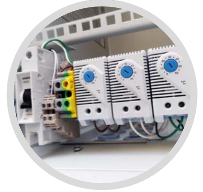
Circuit Breaker and Thermostat
